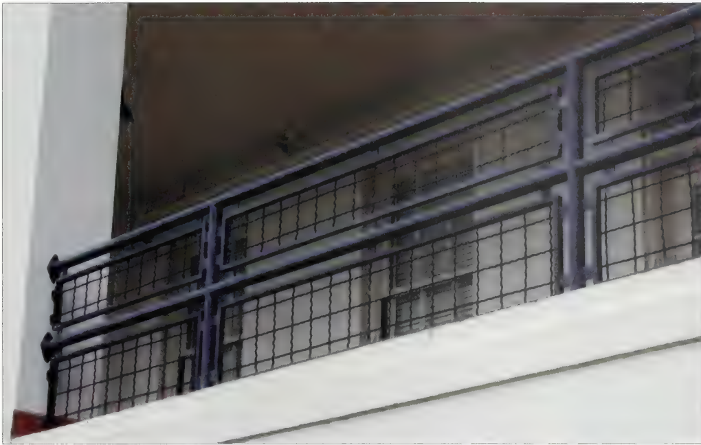
Figure 5.13. Example of the infill approach to retrofitting railing systems for compliance with life-safety codes. In the wide openings between the horizontal pipe rail members, a mesh panel framed by square bar stock has been added. The frame is connected to the existing pipe rails by welding metal tabs between the two (Barbara Judy, Golden Gate National Recreation Area).
